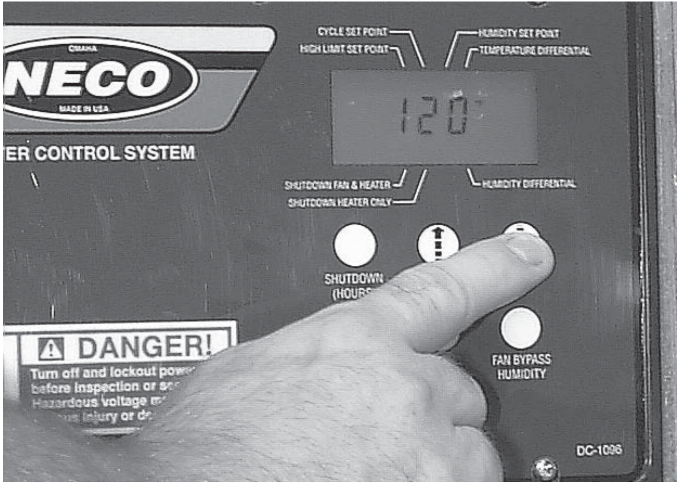
The control panel display showing initial start up.
