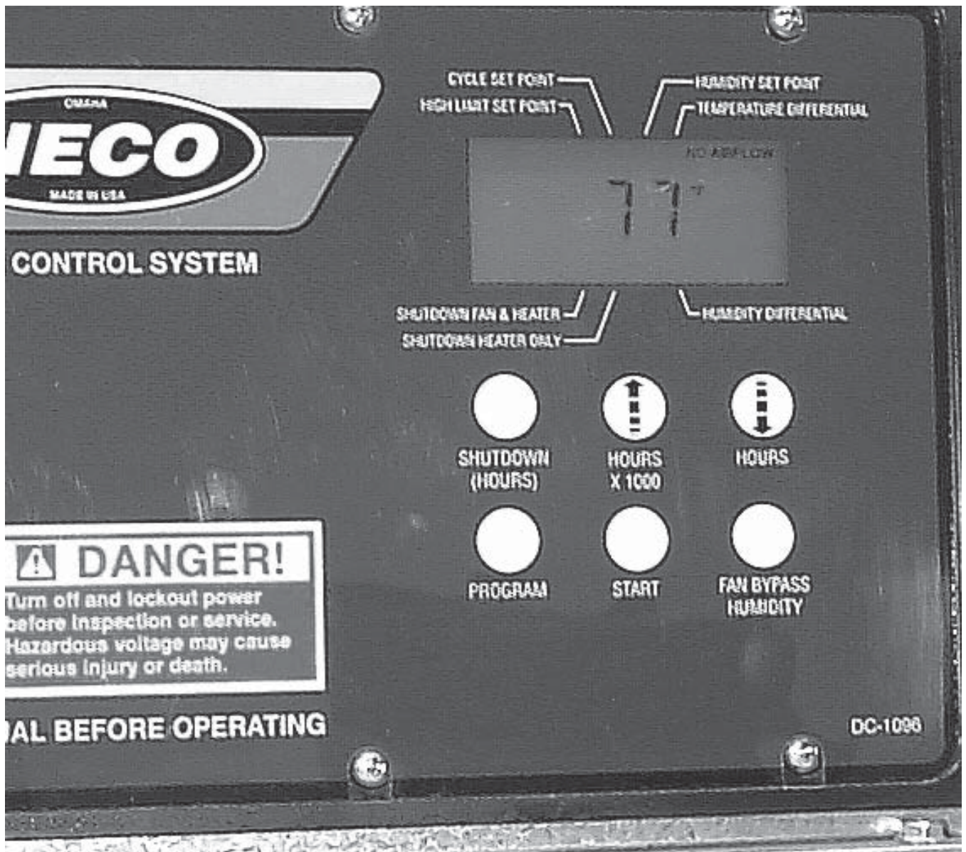
The heater display with fan off ( no airflow).
