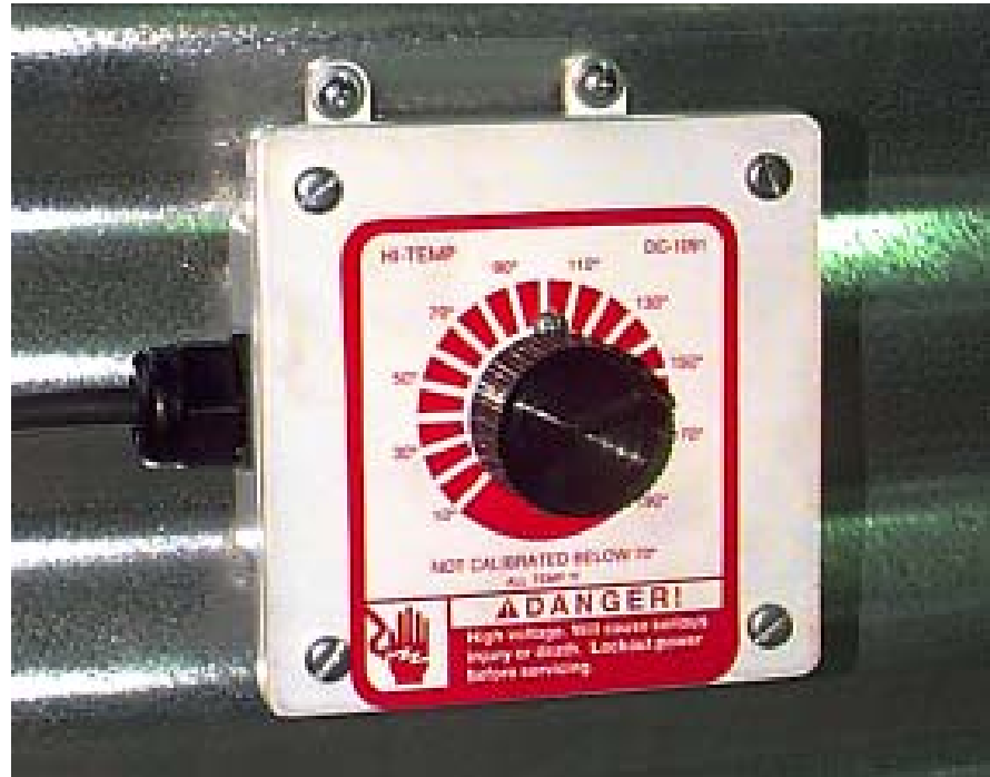
Plenum thermostat mounting on bin wall.
