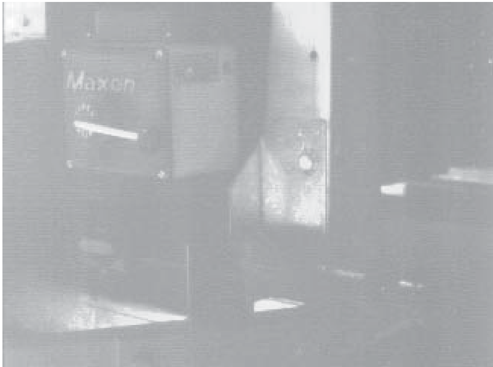
The fuel connection point is equipped with a Y-strainer and Maxon safety valve.
