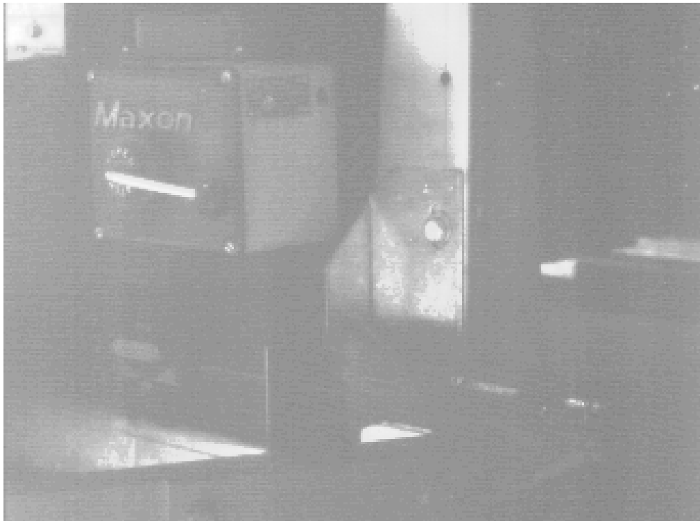
The fuel connection point is equipped with a Y-strainer and Maxon safety valve.
