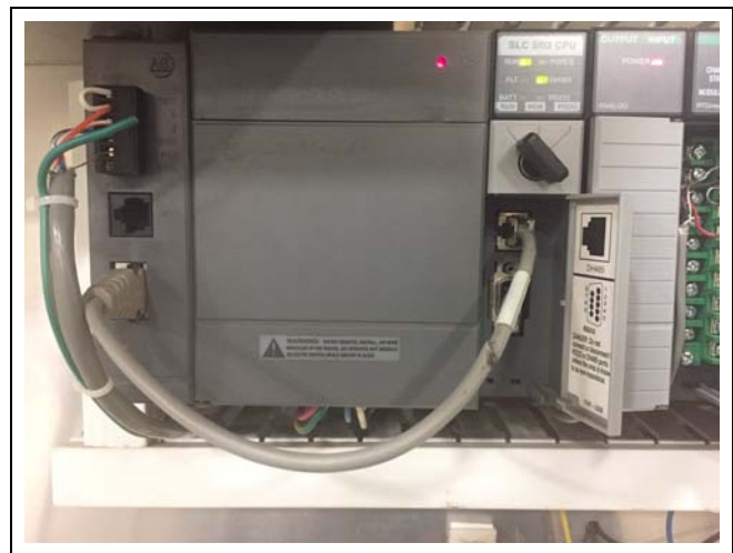
Figure 4 1747-AIC Module Connected to SLC 5/03
