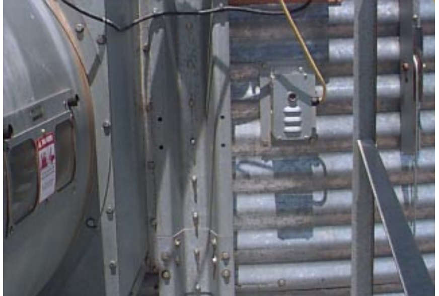
Airswitch mounted on the bin sidewall.
