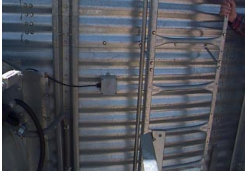
Plenum temperature sensor on the bin sidewall.
