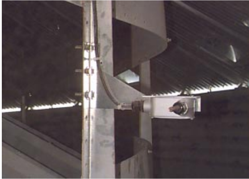
Grain temperature sensor bracket mounted on leveling band post.
