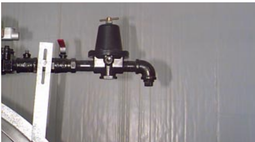
NG line field connection.
