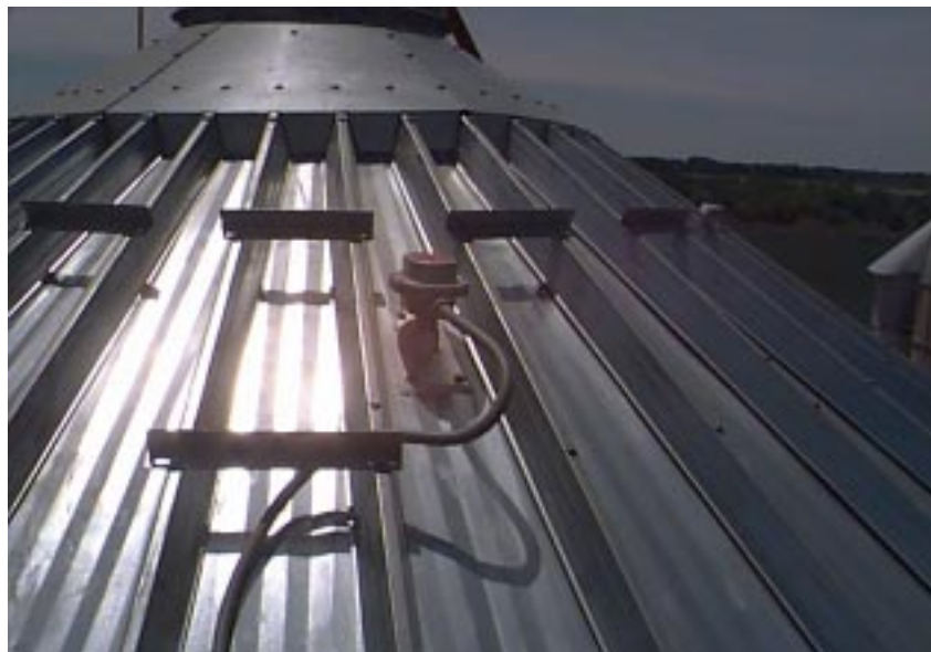
Drying chamber overflow rotary switch.
