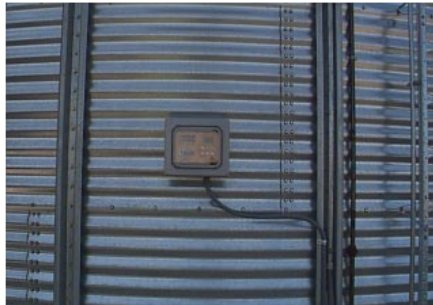
Control box mounted on bin.
