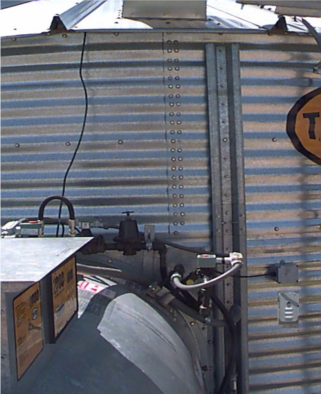
Fan/heater unit mounted to the bin, showing the plenum high limit, the airswitch, and cord going through the eave to the grain temperature sensor bracket.
