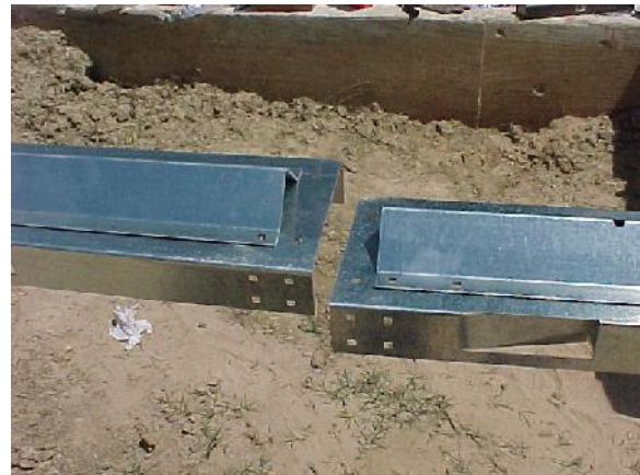
FIGURE 11. BOTTOMS OF THE CHUTES FACING UP
