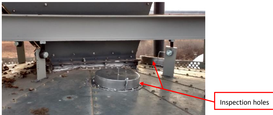
FIGURE 51. SPREADER EYEBOLTS AND SUPPORT ARMS THROUGH ROOF PANELS AND MOUNTED TO CROSS BEAMS
