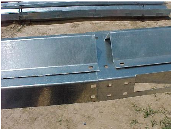
FIGURE 12. BOTTOM CHUTE SLIDING UNDER TOP CHUTE BACK BRACE AT CONNECTION END
