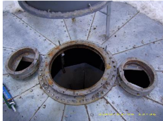
FIGURE 48. INSPECTION HOLES ON COMMERCIAL BIN USING MAXIMUM OPENING
