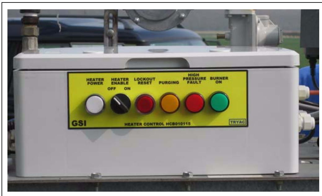
Figure 4K Heater Control Front
