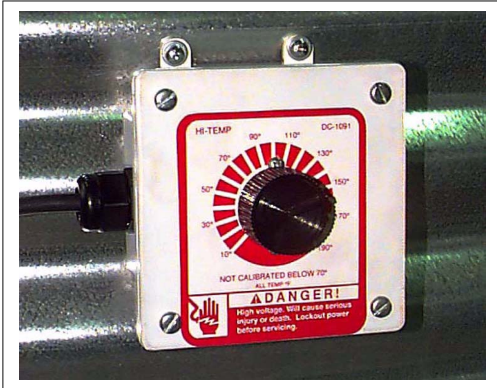
Figure 3E Plenum Thermostat Mounting on Bin Wall
